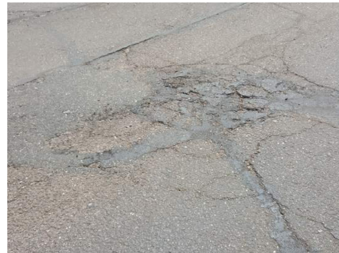
Photograph 12: Low- to medium-severity fatigue cracking, partially sealed, northeast parking area, looking east.
