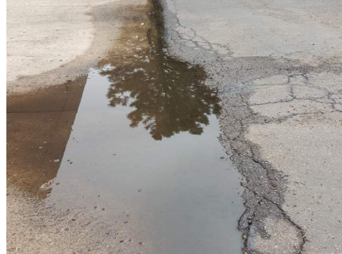
Photograph 6: high-severity edge cracking, fatigue cracking, settlement and ponding, loading dock, looking south.
