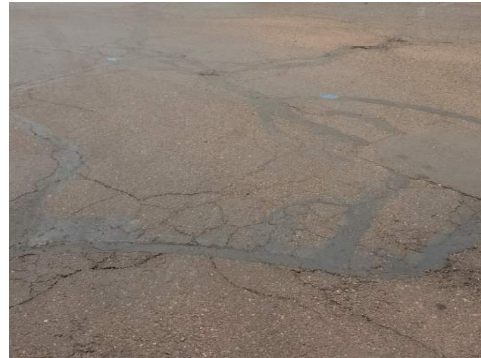
Photograph 8: low-severity fatigue cracking, low-severity raveling, loading dock area, looking south.
