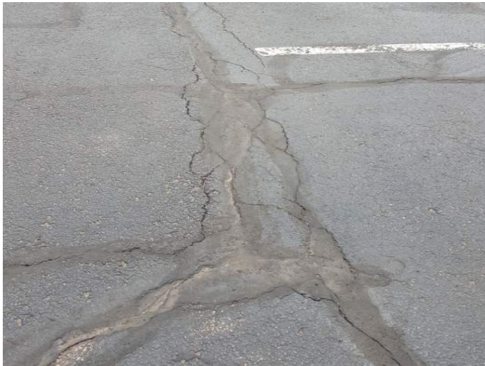
Photograph 13: Low-severity fatigue cracking, partially sealed, lower (west) parking area, looking south.
