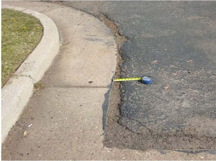
Photograph 9: High-severity edge cracks, low severity raveling southeast parking area, looking north.
