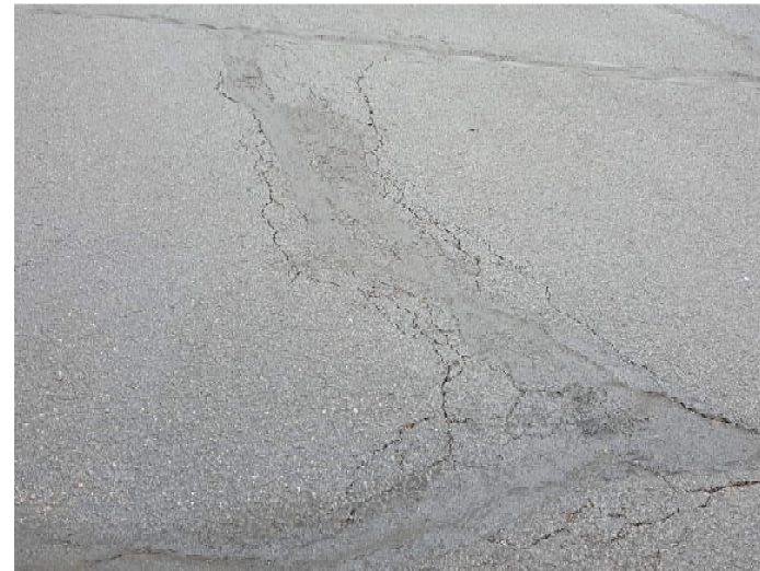
Photograph 14: Low-severity fatigue cracking, partially sealed, lower (west) parking area, looking south.
