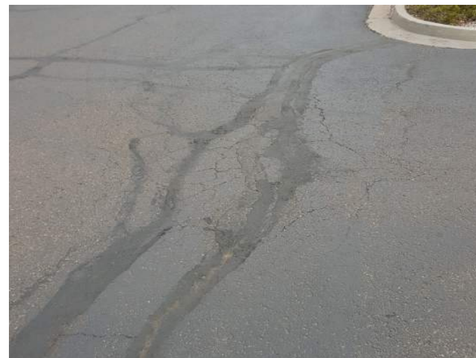
Photograph 16: Low-severity fatigue cracking, low- to moderate severity rutting, south parking area/drive lane, looking east.
