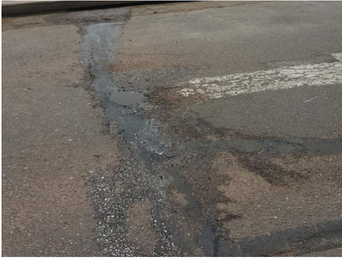
Photograph 1: Moderate- to high-severity cracking and ponding in main entrance, looking south
