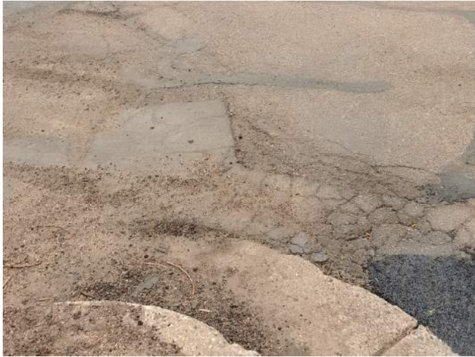
Photograph 5: Low- to moderate-severity fatigue cracking, and patches, loading dock, looking southwest.
