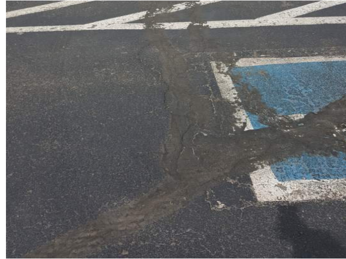
Photograph 2: Partially sealed moderate-severity fatigue cracking, main entrance ADA parking, looking west.
