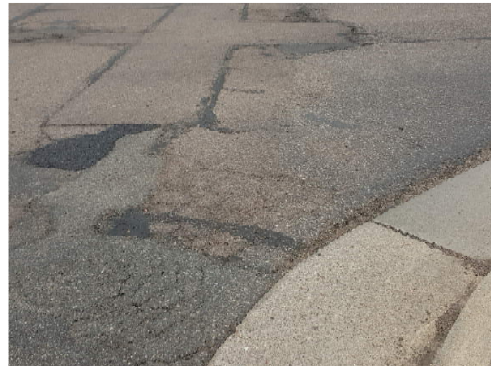
Photograph 4: Low-severity fatigue and joint cracking around patches, SW entrance area (Area No. 2), looking north.
