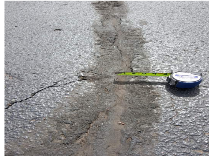
Photograph 10: Sealed high-severity transverse cracking, southeast parking area, looking east.
