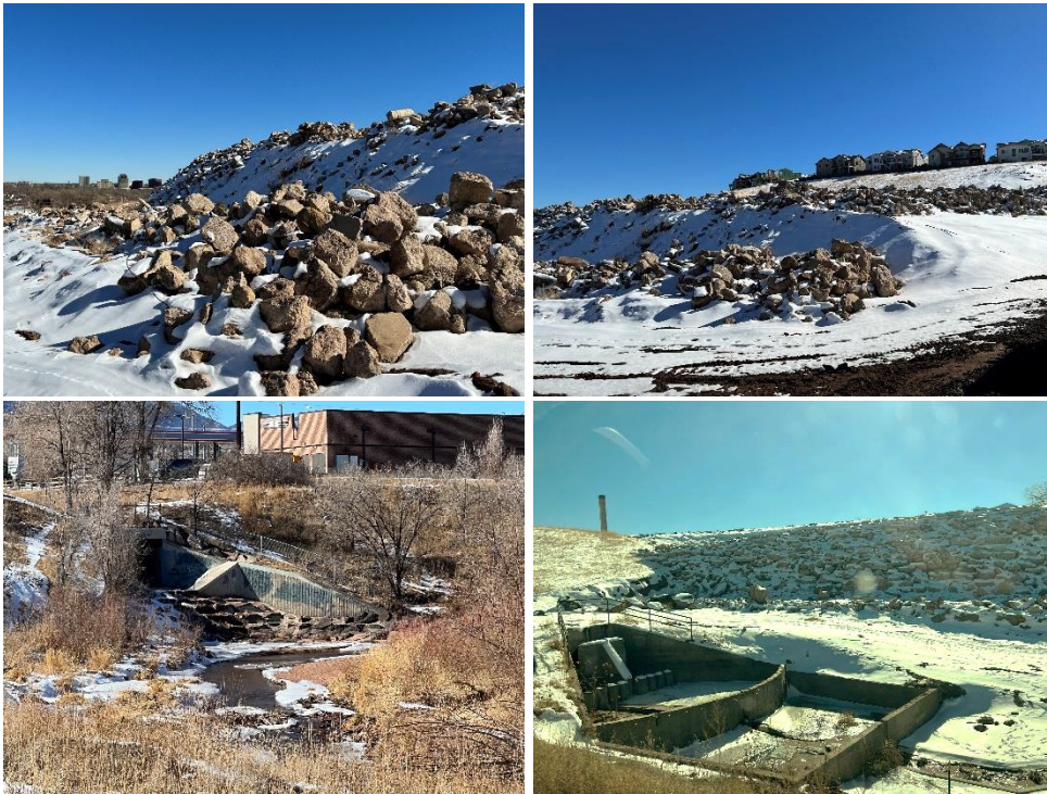
Figure 8. Inadequate Storm Drainage System
