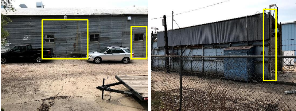
Figure 2. Deteriorated Exterior Finishes and Ancillary Structures
