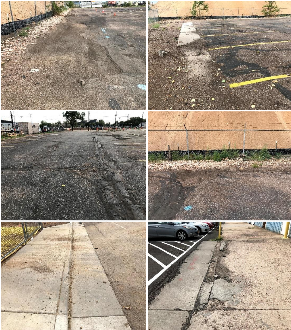
Figure 8. Deteriorated On-Site Parking Surfaces, Curb, & Sidewalks
