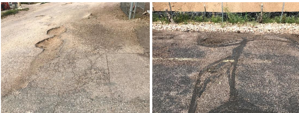
Figure 10. Deteriorated Pavement, Curb, and Sidewalks
