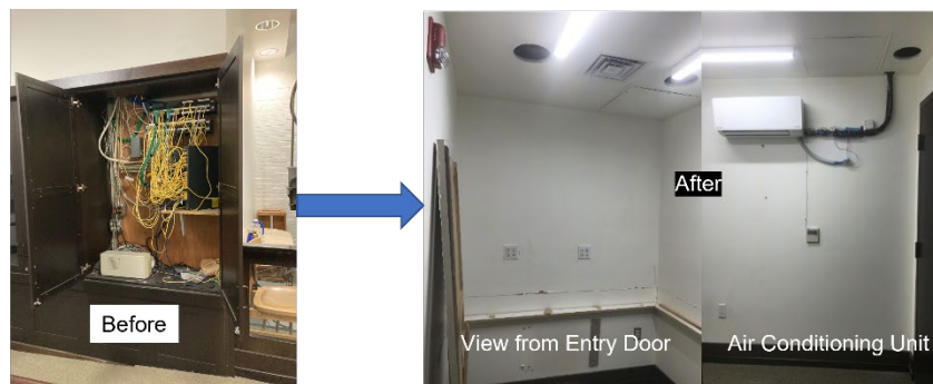
Transition from “closet” to intermediate distribution frame room to accommodate PE cabling project.
