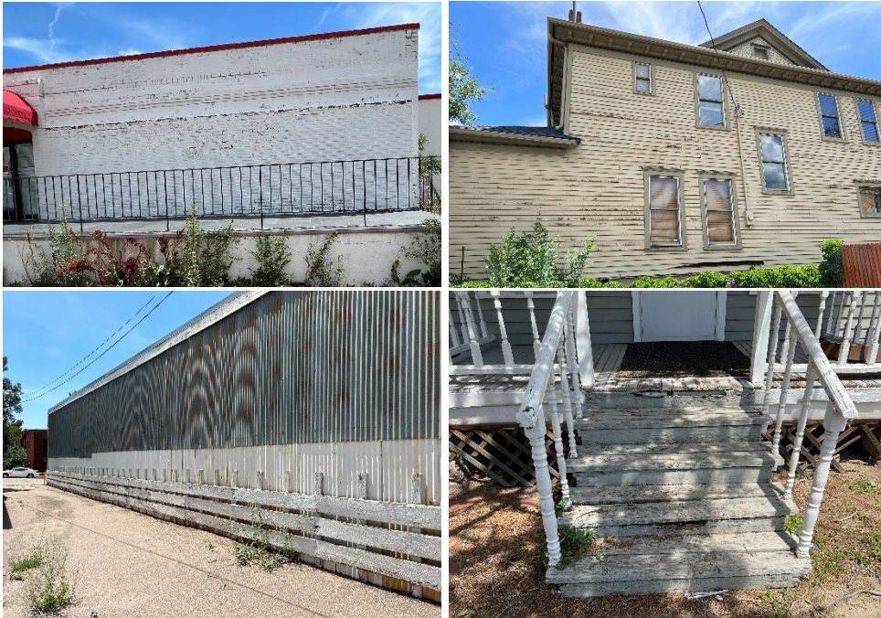
Figure 2. Deteriorated Exterior Finishes and Stairways
