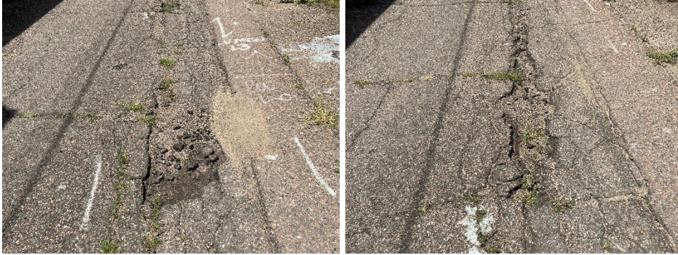
Figure 4. Poor Provision of Street Improvements for Vehicles
