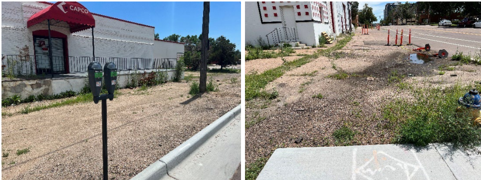
Figure 13. Lack of Sidewalks and Curb
